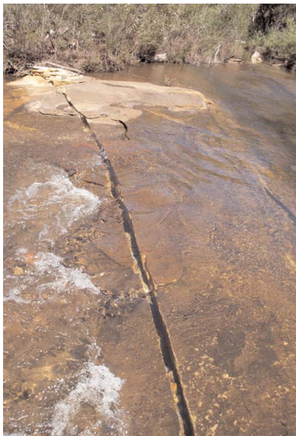
Cracking of the Waratah Rivulet bed, in Sydney catchment area
